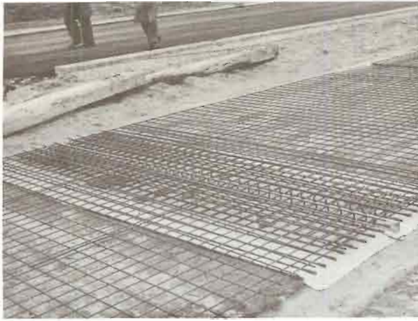
Figure 53. General view of the tendons, transverse reinforcement, hairpin reinforcement, etc. at a transverse joint. (See also Figure 45.)
