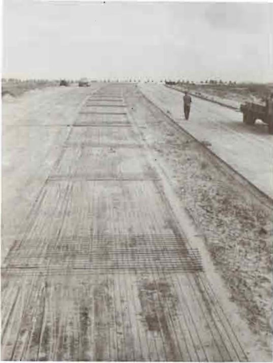
Figure 49. General view of prestressed road with tendons (some of which are already tensioned) and transverse mesh reinforcement.
