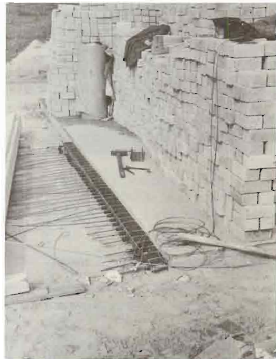
Figure 52. Abutment with kentledge of stacked blocks; the anchorages of the tendons are distinctly visible.
