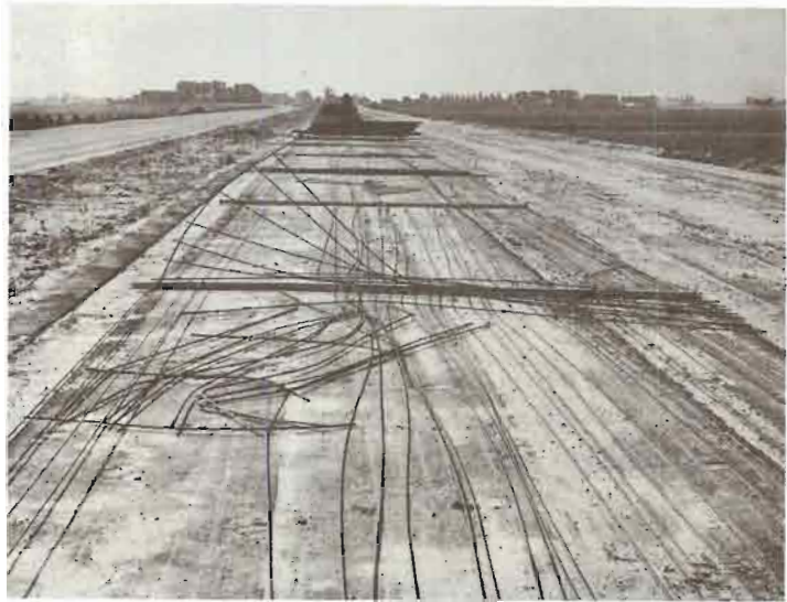
Figure 50. Havoc caused by a fractured tendon
